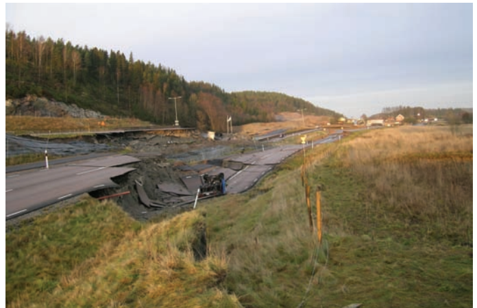
Figure 13 Munkedal landslide (2006) affecting the Oslo-Gothenburg traffic.
