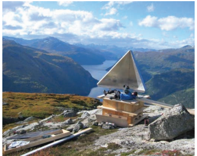
Figure 6 Installation of radar reflectors for monitoring movements of unstable mountains in Storffjorden, western Norway. Rockfalls into fjords and lakes may create large tsunamis that will damage the settlements and infrastructure (Photo: Lars H. Blikra).
